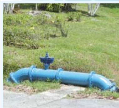
One of the numerous water pipes that could potentially be damaged during water theft
